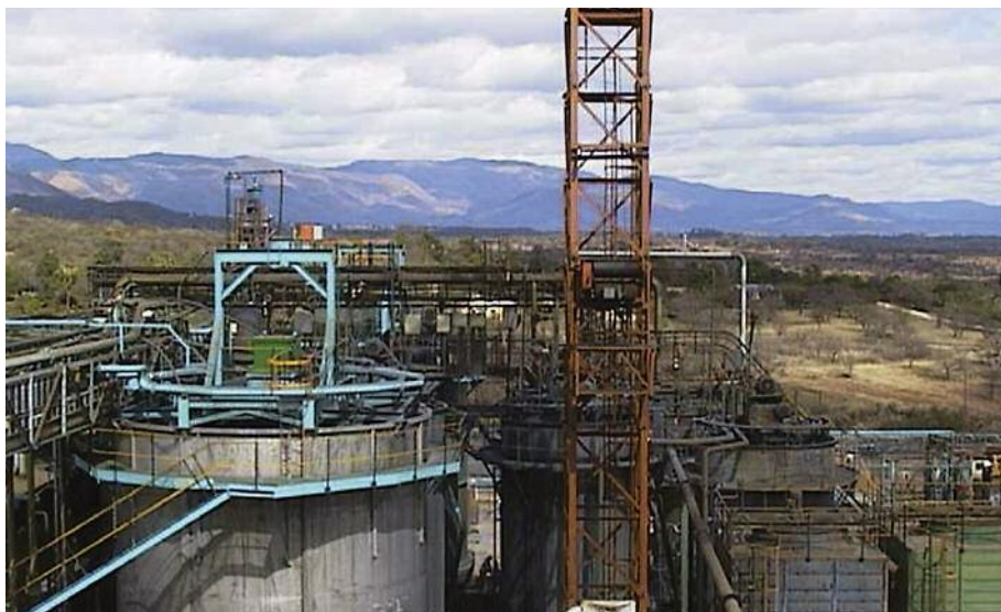
The Fairview BIOX® Plant.
